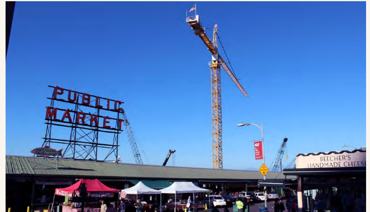
On October 15, 2015, a crane was installed to begin the heavy construction on the MarketFront expansion. (Emily Crawford, PDA)
