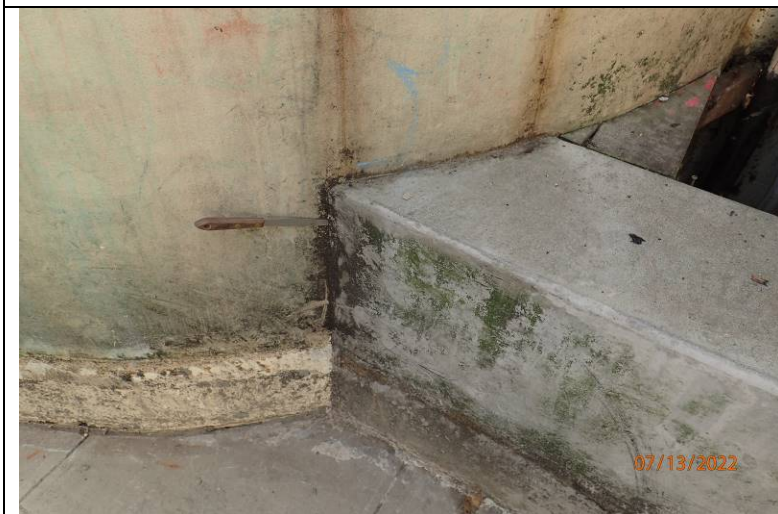
Photograph 18: Sealant knife inserted into open joint between the curb and round structure at the stairs. This joint should be sealed.
