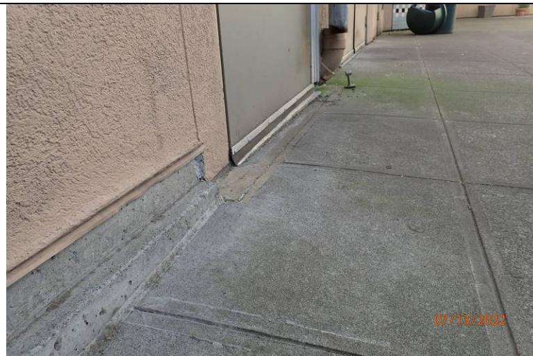
Photograph 14: Looking west along the north wall of the Heritage House. The door in the photo is to the hallway in photos 10 & 11. Note the concrete curb in the left of the photo, which is not present west of the door.
