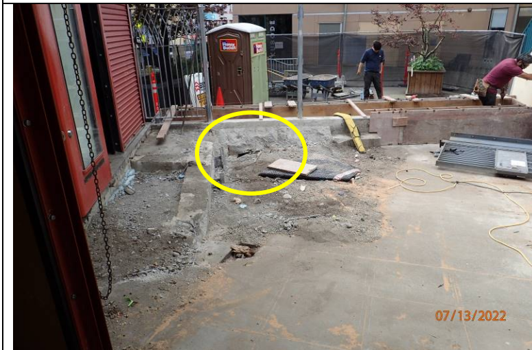
Photograph 20: Looking south at the concrete stem wall and existing drain mat (circled) found that travels under the wall.
