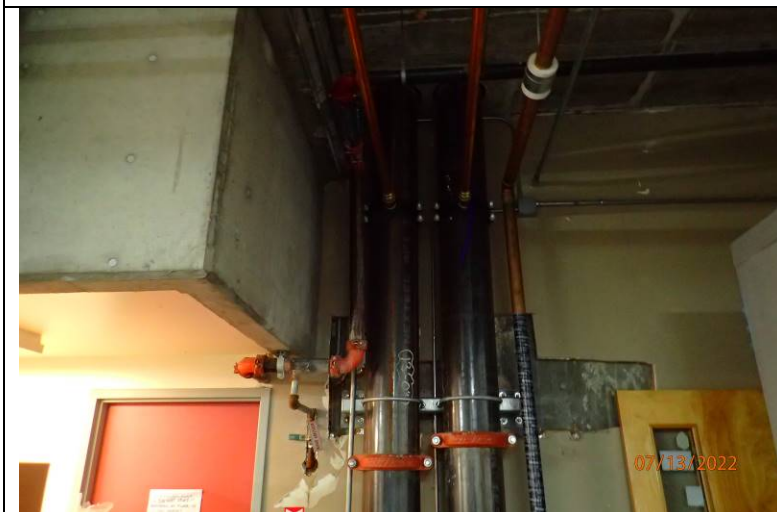
Photograph 24: Chiller lines within the garage/food bank space, below the north side of the elevators.
