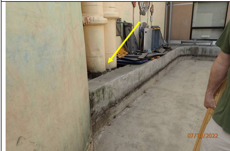
Photograph 17: The curb in the photo is over the plaza topping slab, it appears, and has weeps at the bottom. The weeps were reportedly clogged and water becomes trapped on the south side of the concrete curb (arrow). Weeps should be cleaned and maintained so they remain open to drain.
