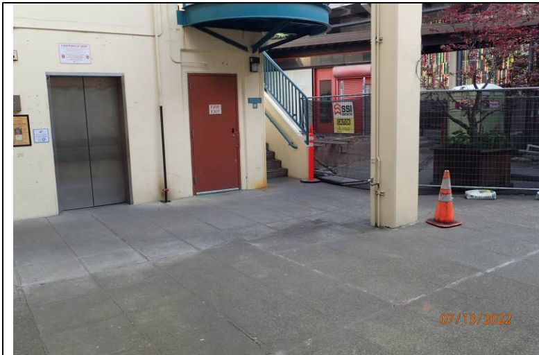
Photograph 4: Looking north and east at the elevator shaft and area of construction at the north by SSI.
