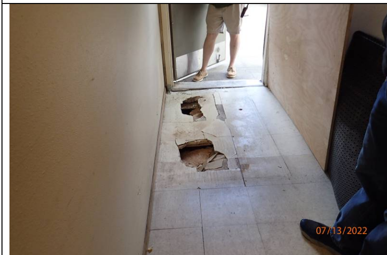
Photograph 9: Looking north at the damaged floor to the east of Stairwell B. Reportedly, the floor caved in when moving heavy carts over the surface.
