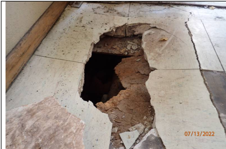
Photograph 10: Closer view of the damaged floor. It appears the substrate has deteriorated, likely due to moisture within the assembly.
