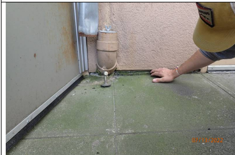
Photograph 12: Looking at the plaza-to-wall transition outside the hallway in the previous photo, further west. Note the downspouts were disconnected from the below grade drain lines and allowed to discharge onto the plaza, which reportedly has reduced leakage into the garage below.
