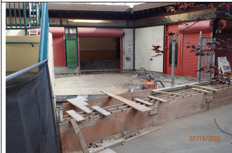
Photograph 6: Area of construction by SSI, showing form work for new concrete walls.
