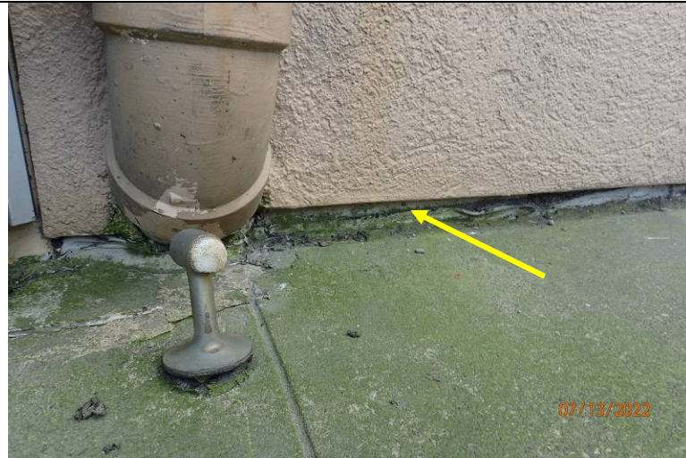
Photograph 13: Closer view of the previous photo. The substrate below the stucco and above the plaza topping slab appears to be sheathing covered with metal, and not concrete.
