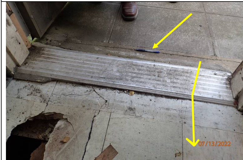
Photograph 11: Where the pen is placed appears to be the top of a concrete stem wall that separates the plaza from the Heritage House exterior wall. The top of the stem wall is exposed and could allow water under the threshold and into the floor cavity.
