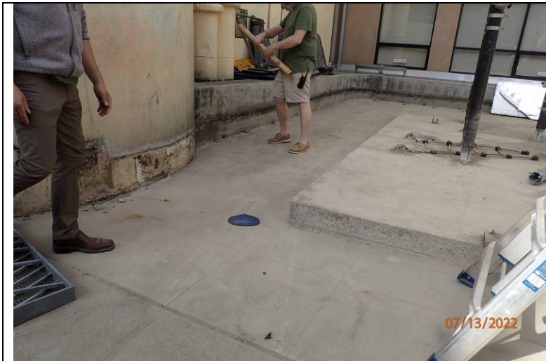
Photograph 16: Looking west at the north side of the round stairwell structure and elevator shaft structure at the west side of the plaza.
