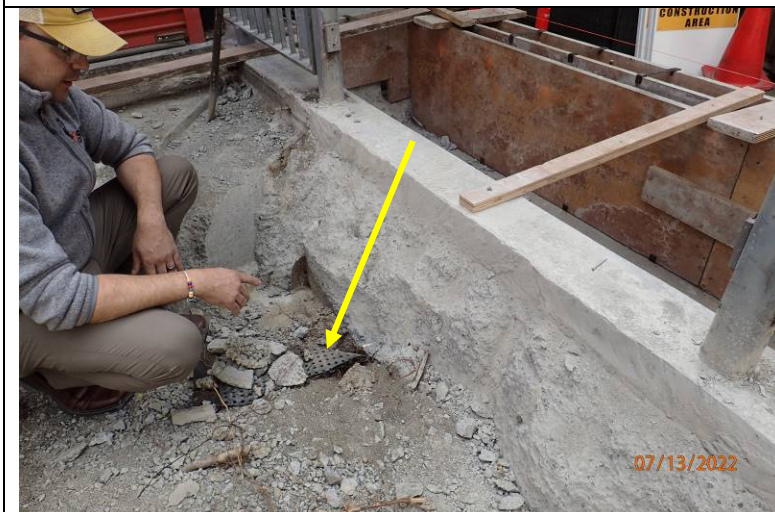
Photograph 21: Closer view showing the drain mat. We understand this wall will be removed to allow new drain mat installation.
