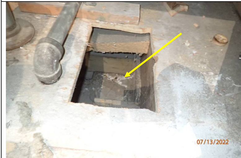
Photograph 8: Looking inside the access area in Stairwell B. Note the water stains on the concrete substrate below the wood framed floor. Water entry has occurred under the wood framed flooring on the lid of the garage below.
