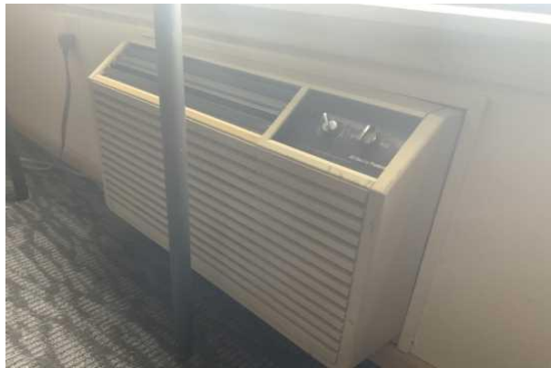
28 THRU WALL A/C UNIT
