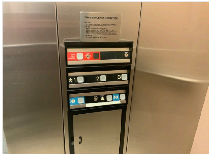
In-cab controls/emergency call panel
