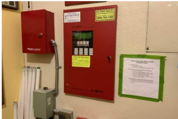
22 FIRE ALARM SYSTEM
